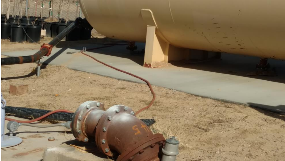
Maintenance Yard Area looking at Agricultural Well - Unused Connection
